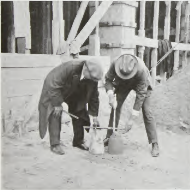
Association fieldman assisting contractor with slump test to determine right consistency of concrete.
